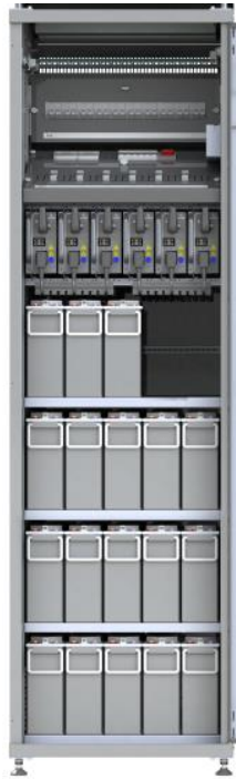
OPUS HE 220-12.0 OC2066 220VDC 9.3A – 55.5A 2 x MCB 63A battery fuses Battery & distribution space
