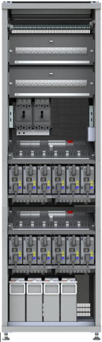
OPUS HE 24-18.0 OC2066 24VDC 62.5A – 750A 2 x MCCB 460A battery fuses Battery & distribution space
